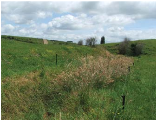
A weed choked drain.
