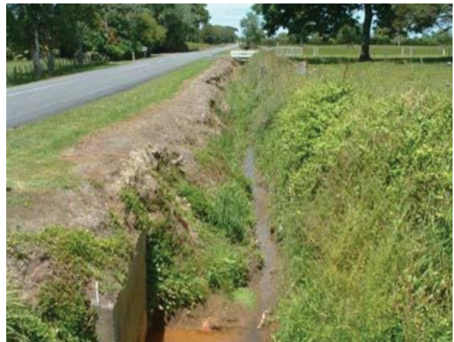
Bank erosion resulting from spraying the drain edge.
