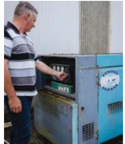
Greg (pictured with the farm's generator) says an alternative power source is a "must-have".
